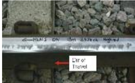
Figure 1a: RCF on a shallow high speed curve. The cracks are high on the gauge shoulder and crack directions are traversing the rail head.
