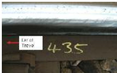
Figure 1b: RCF on a sharp slow speed curve. The cracks are near the gauge corner and crack directions are more parallel to the running rail.
