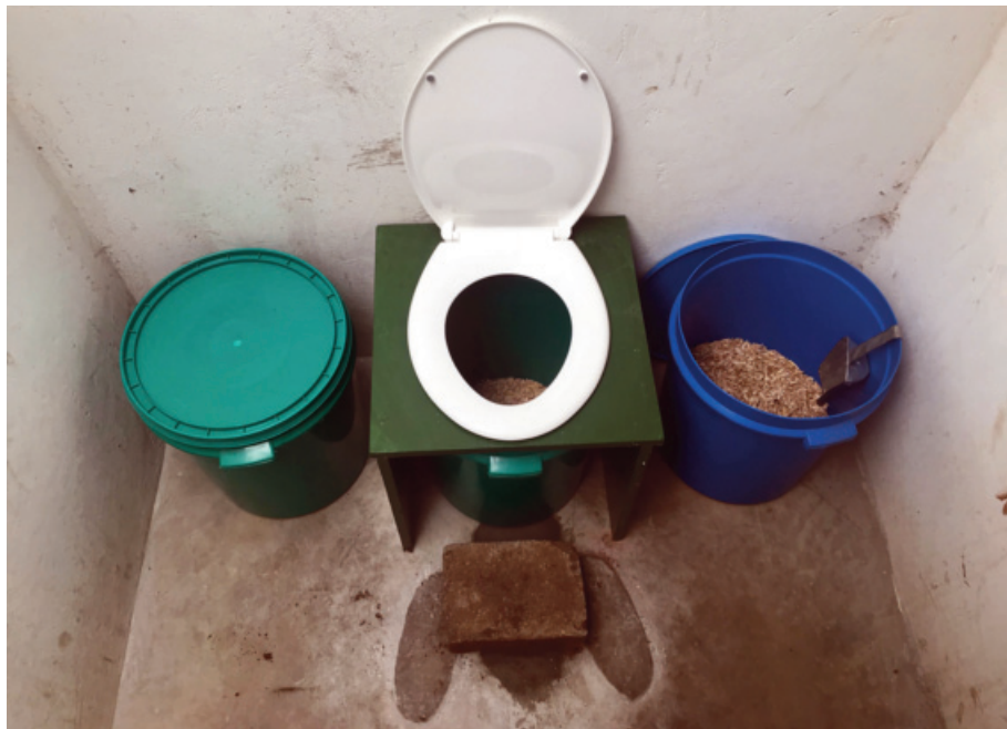
This is a pit latrine converted into a compost toilet at the Police Academy children's school in Moroto county, Karamoja, Uganda (a WeltHungerHilfe project).
